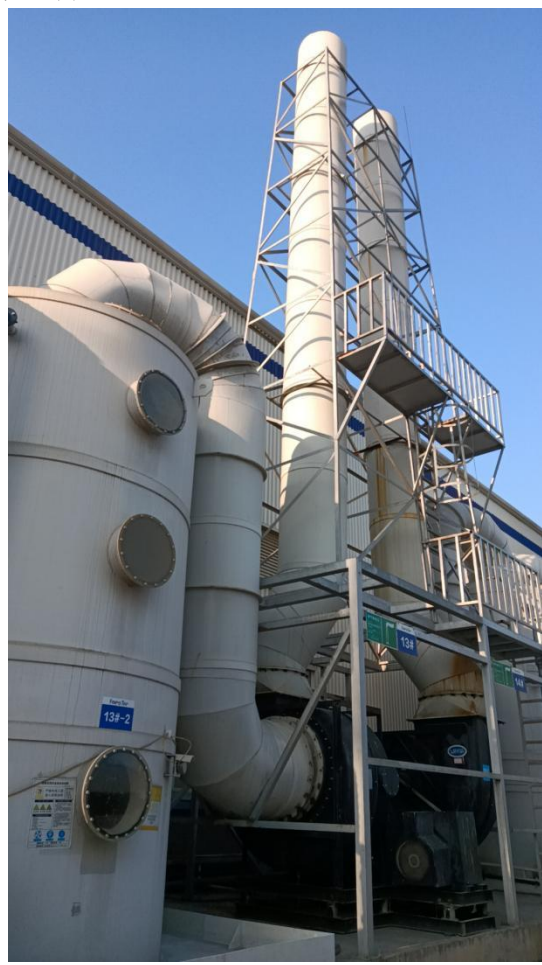
碱洗+氨水浸泡废气排气筒
