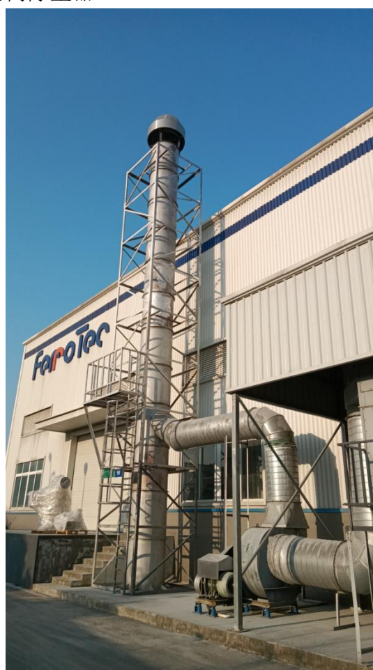
DA011 喷砂粉尘排气筒
