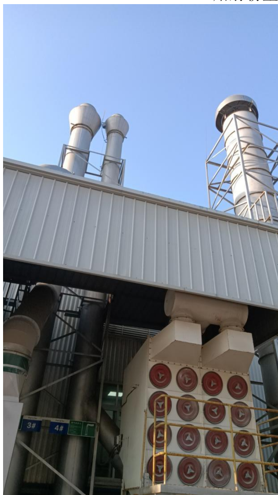
DA014、DA015 熔射粉尘排气筒
